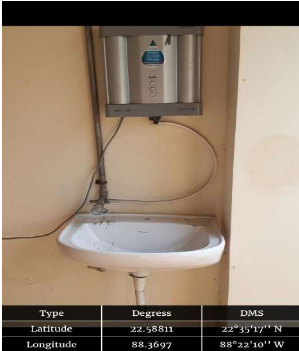
Water purifier at Jubilee Bld (2 nd Fl.)
