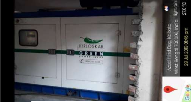
GENERATOR AT PREMISES NO 1
